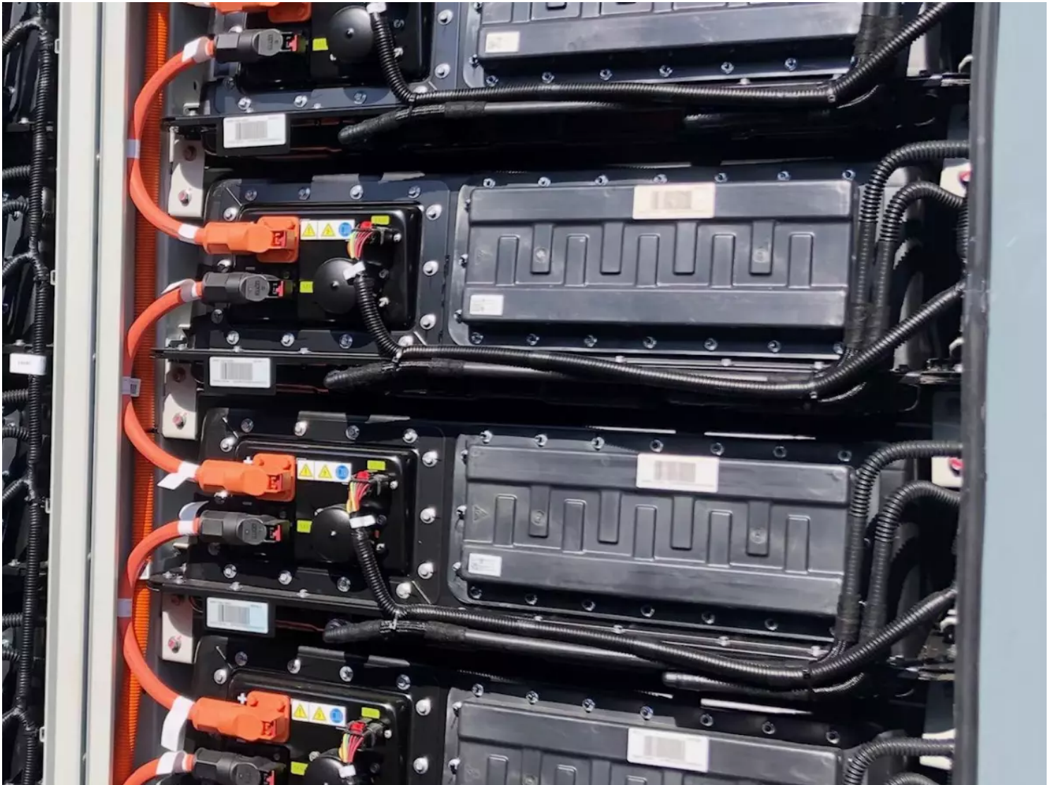
Closeup of batteries inside one of the cubes at the SDG&E Kearny Energy Storage battery storage facility in Kearny Mesa. The project delivers 20 megawatts and 80 megawatt-hours of electricity to California's grid. (Rob Nikolewski/San Diego Union-Tribune)
